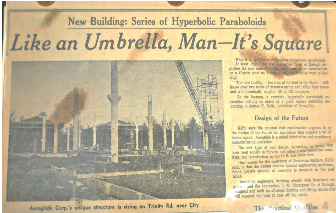
Figure 3. Aeroglide Corporation Building Under Construction. Source: News and Observer (Raleigh, North Carolina), February 23, 1964.
